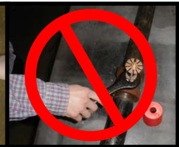
INCORRECT! (sprinkler at floor level)
