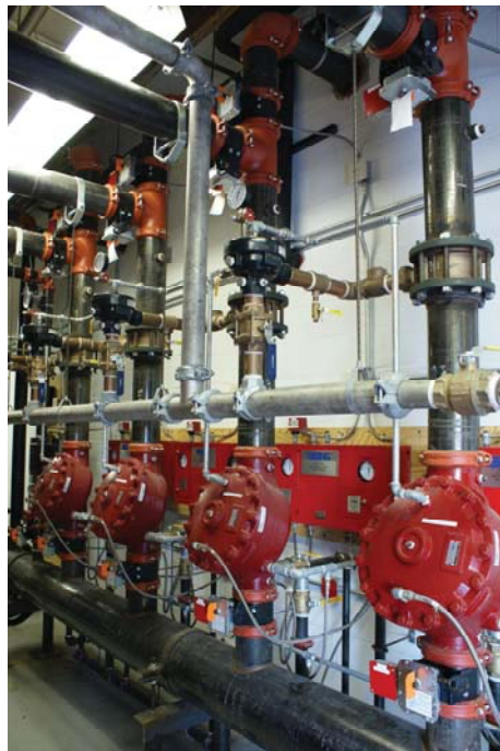
Figure 1: Foam Deluge Riser – Photo Courtesy of S&L Mechanical
