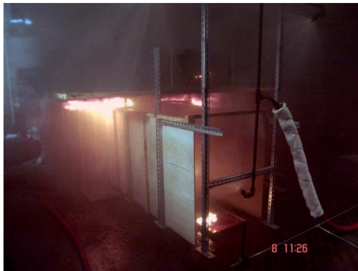
Figure 4: Fire test shortly after activation of the fine water spray system
