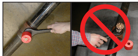
CORRECT (Piping is in place at the ceiling)
