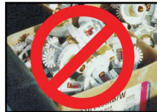
INCORRECT (Protective caps not in place)
