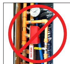
INCORRECT (No pressure relief valve)
