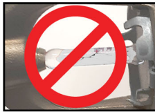
INCORRECT (bulb cracked, fluid missing)
