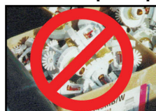
INCORRECT (Protective caps not in place)
