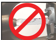
INCORRECT (bulb cracked, fluid missing)
