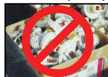
INCORRECT (Protective caps not in place)
